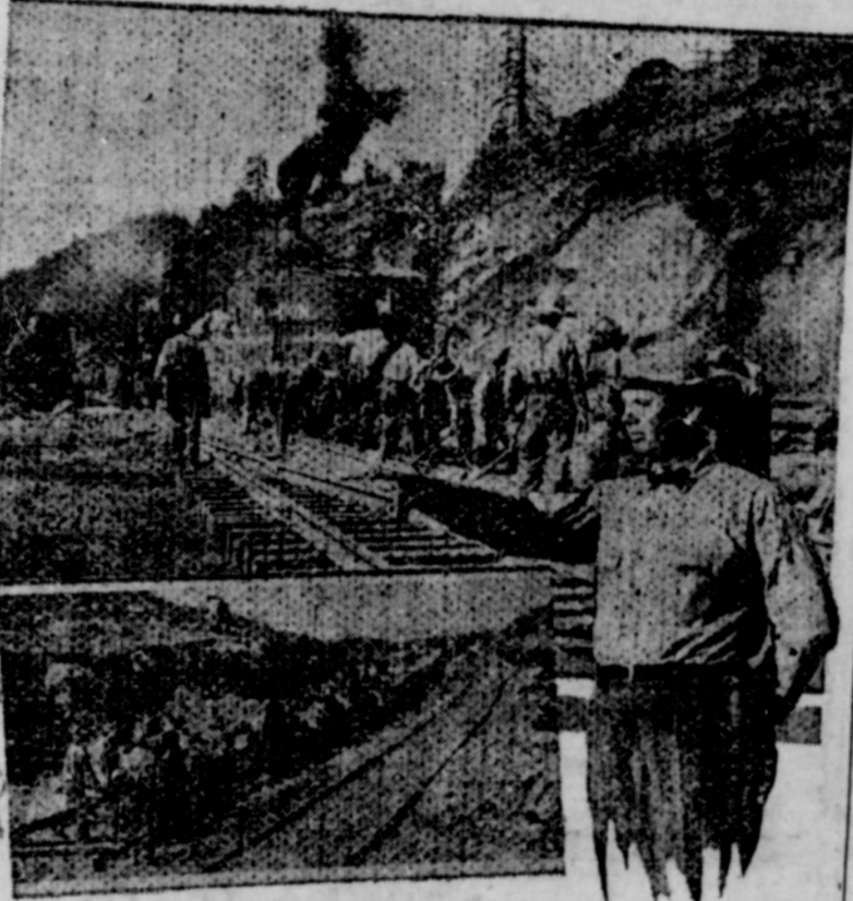
Above is shown one of the many gangs of workmen using steam shovels and other equipment to open the way through the famous Emigrant Gap for additional trackage. (Below) Track laying crew setting a last stride between Montello and Loran in Nevada. Engineer Otis Weeks directing important construction work.
