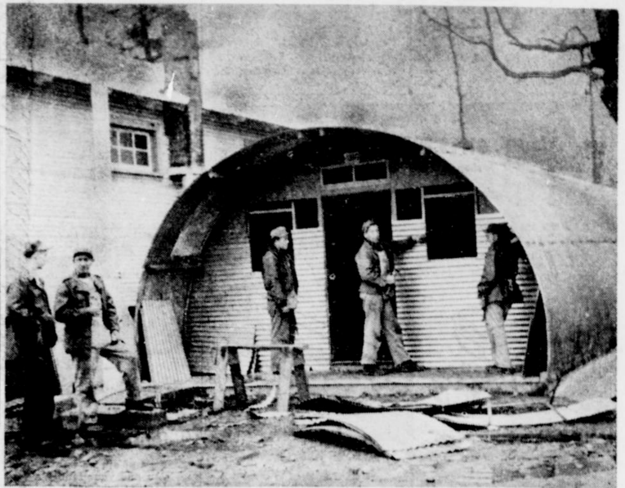
Lt. Otis Hussey talks to Sgt. Robert Houghton, in charge of erection of local national guard building. Men in background are putting finishing touches on quonset. —ILLINOIS VALLEY NEWS PHOTO
