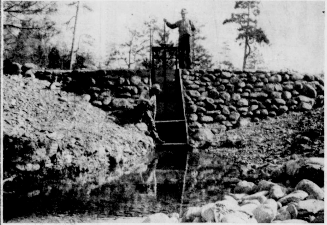
Farmers Russel Doran (sitting) and C. E. Burton (standing) survey the new gate and headworks they built this summer for a year-round irrigation
