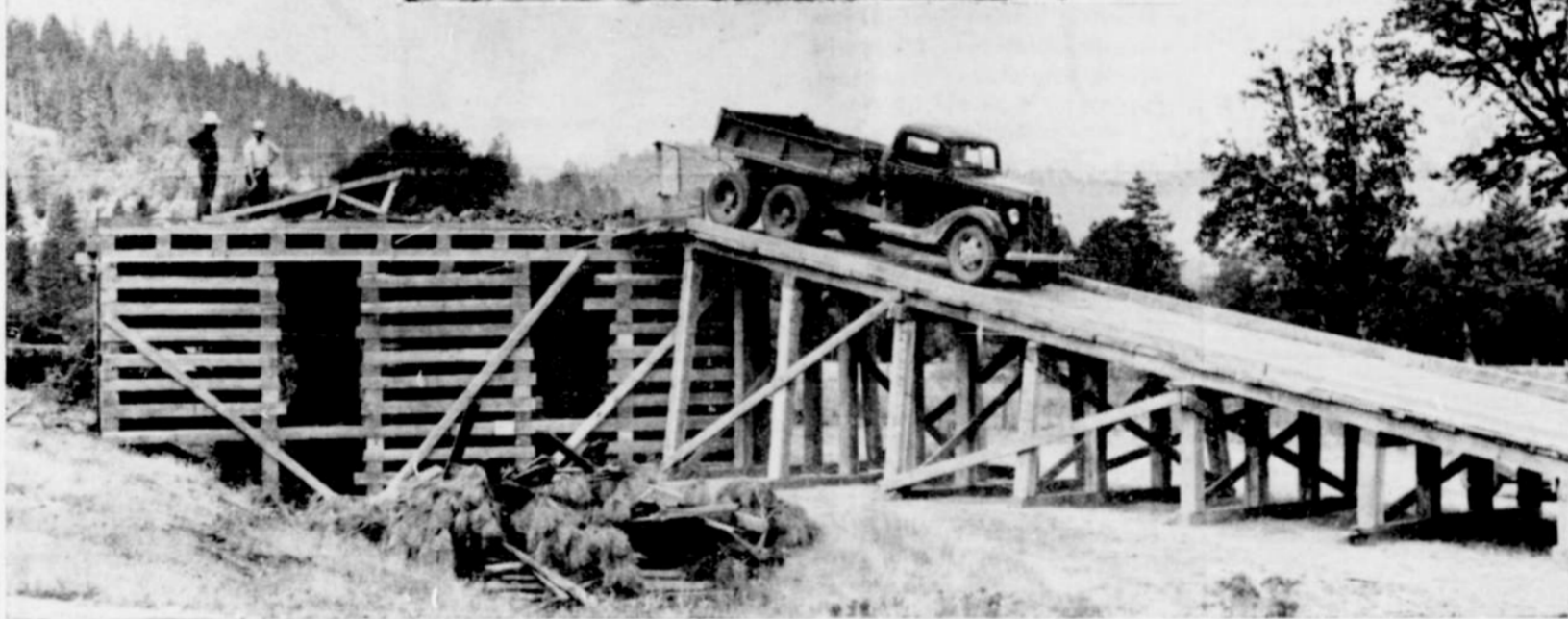
This loading platform built at Wilderville to load 2000 tons of chrome ore for the American Rustless Iron and Steel Corporation of Baltimore, Maryland, is swelling freight traffic over Grants Pass municipal railroad, the California & Oregon Coast line. The chrome, hauled in continuous 8-hour round trips from High Plateau in northern California beyond O'Brien at Eugene Brown's mine by the truck shown in the photo below, is backed up the incline to the elevated bunkers from which it is dropped into railroad gondola cars below. At top, J. E. Bartlett (left) and J. E. Hutcheson watch a truckload of ore dumped. Chrome from other mines is moving to other shipping points at Grants Pass, Glendale and Medford.—Cut courtesy of the Grants Pass Courier.
