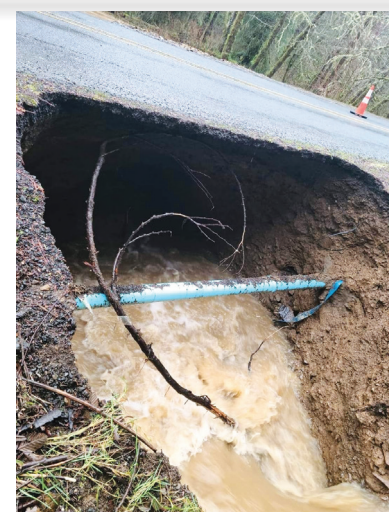
Flood water erodes the base under Highway 202 in Astoria.
