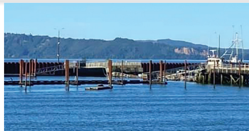
A 250-foot section of the East Mooring Basin Causeway collapsed.
