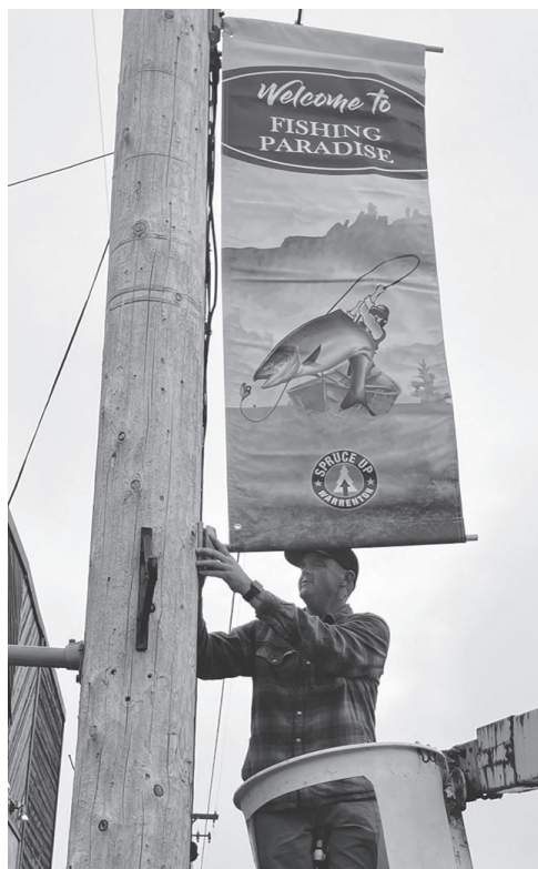
Fire Chief Brian Alsbury uses a bucket truck to help Spruce Up install its new summer banners along Main Avenue.
