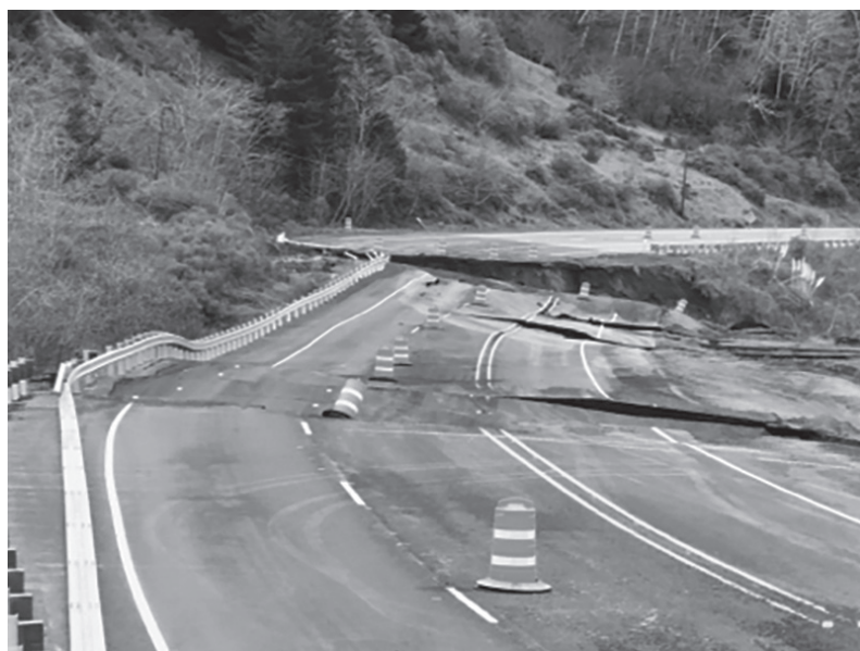
Oregon Department of Transportation The Hookskanaden Slide near Brookings moved across Highway 101 in March 2019, disrupting traffic for several months.
