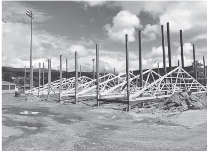
Roof trusses and framing are going up at an indoor athletic facility at Broadway Park in Seaside.
