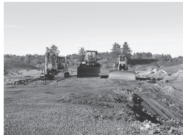
Top left: Earthmoving equipment stands at the ready Wednesday morning at a development off Highway 101 in Clatsop Plains.
