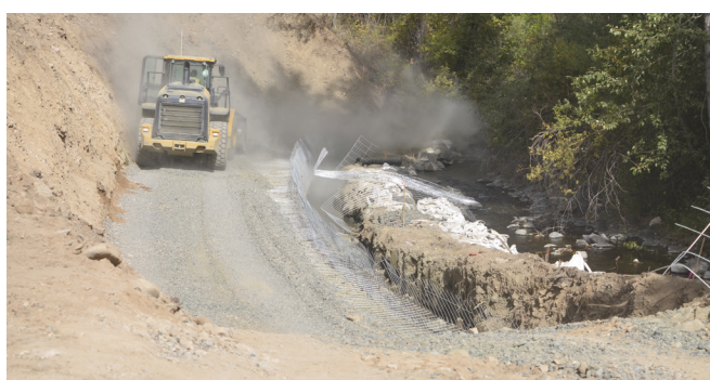
Justin Davis/Blue Mountain Eagle Lee Duckett of Tidewater Contractors operates a front loader on Wednesday, Sept. 29, 2022. The company is shoring up a flood-damaged portion of Southwest Fourth Avenue in John Day.
