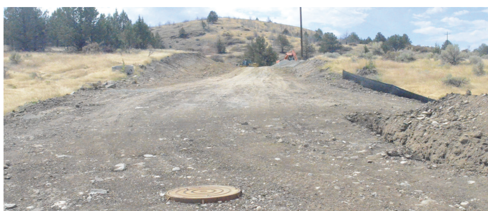
Am unpaved road with manhole installed at The Ridge on Monday, Aug. 8, 2022.
