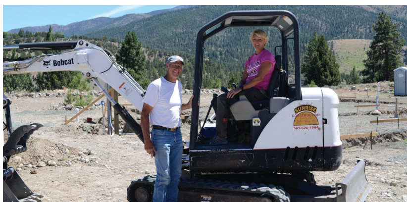
Justin Davis/Blue Mountain Eagle Bruce and Kimberly Ward on the site of a new home lot they're developing at Canyon Mountain Heights in Canyon City on Monday, July 11, 2022.
