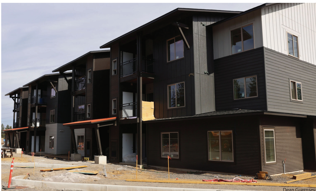
The Stillwater Crossing affordable housing apartments under construction at the south end of Bend in October.
