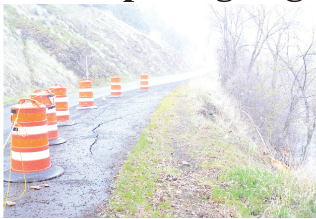
The damaged road and eroded embankment on Southwest Fourth Avenue in John Day. The road has been in need of repairs for almost three years.
