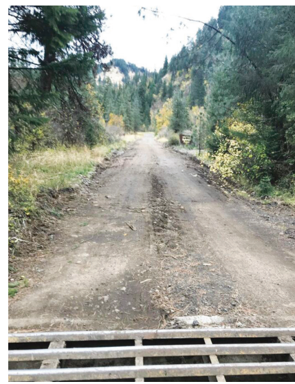
Umatilla National Forest/Contributed Photo A section of Road 32 on the Umatilla National Forest near Umatilla Forks campground has reopened following repairs to sections damaged by flooding in February 2020.
