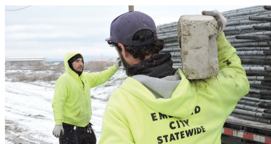
Erick Peterson/East Oregonian Tony Castro and Jason McCary of Emerald City Statewide set up fencing on Thursday, Feb. 24, 2022, around the wreckage of Shearer's Foods, Hermiston, two days after an explosion and fire destroyed the facility.
