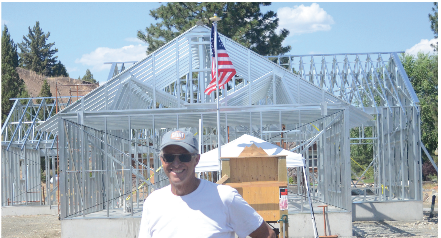
Steven Mitchell/Blue Mountain Eagle Bruce Ward stands in front of a steel-framed house under construction. Ward, who owns Sunrise Construction Specialties, is a longtime evangelist for the fire-resistant construction technique.
