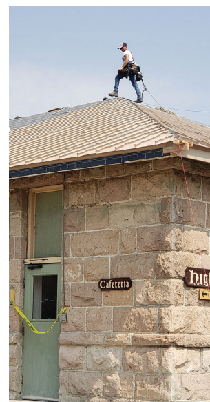
Contributed photo Dayville Superintendent Kathryn Hedrick said repairs to the school's roof and awnings are almost finished.
