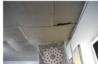
Sagging ceiling tiles caused by leaks at a Boring Properties unit in John Day.
