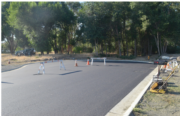
The Eagle/Rudy Diaz The first cul-de-sac in John Day on the northern end of Northwest Canton Street will be near parking for the new Hill Family Park, which will provide access to the John Day River.
