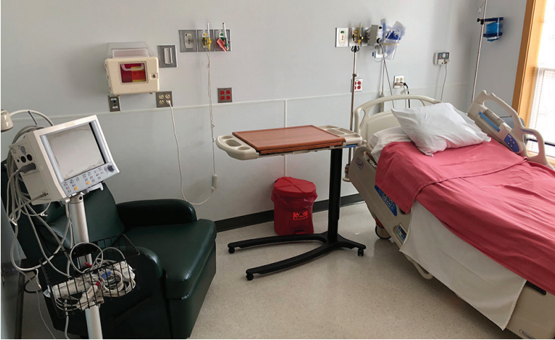
Contributed photo A permanent negative pressure isolation room at Blue Mountain Hospital. The hospital has three negative pressure rooms available for isolation:
