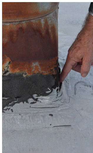
Grant County Court Judge Scott Myers shows why the roof needs to be replaced at the courthouse and why leaks happen.
