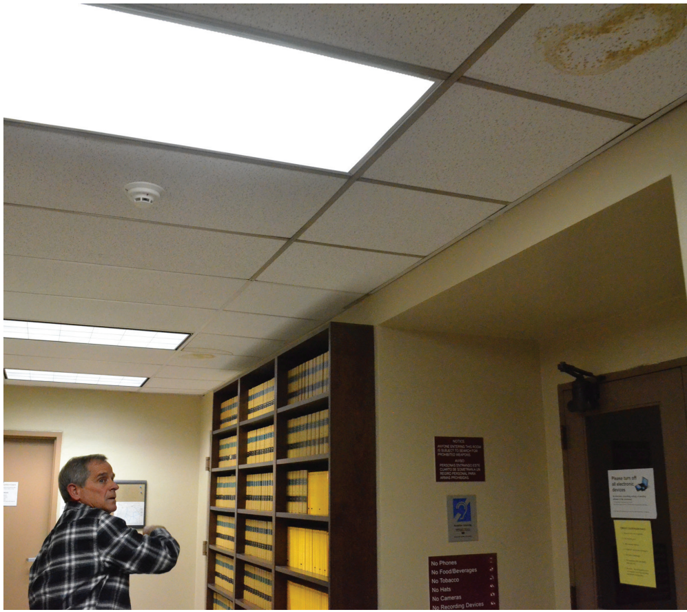
Judge Scott Myers pointing at the various leaks on the third floor of the Grant County Courthouse.
