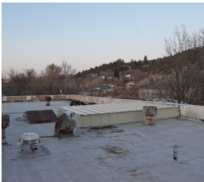
A majority of the fans on the roof will be taken out since they are old and have been the source of many leaks.
