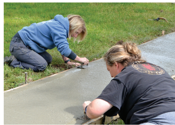
The Eagle/Angel Carpenter Monument teacher Michele Engle and parent and city council volunteer Heather Bowlus help with the edging of the park sidewalk.
