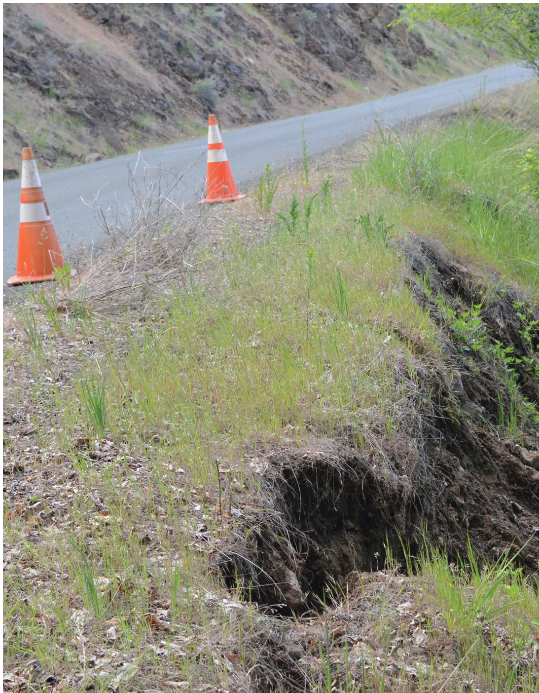
The Eagle/Richard Hanners Recent flooding in Canyon Creek eroded the steep embankment on Fourth Avenue Southwest leading to the Grant County Regional Airport creating a serious road hazard.
