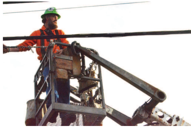
The Eagle/Richard Hanners A Blue Mountain Telecommunication Services worker on a bucket truck helps run an optical fiber cable along South Canyon Boulevard from the John Day Fire Hall to the Grant County Education Service District building on April 3.
