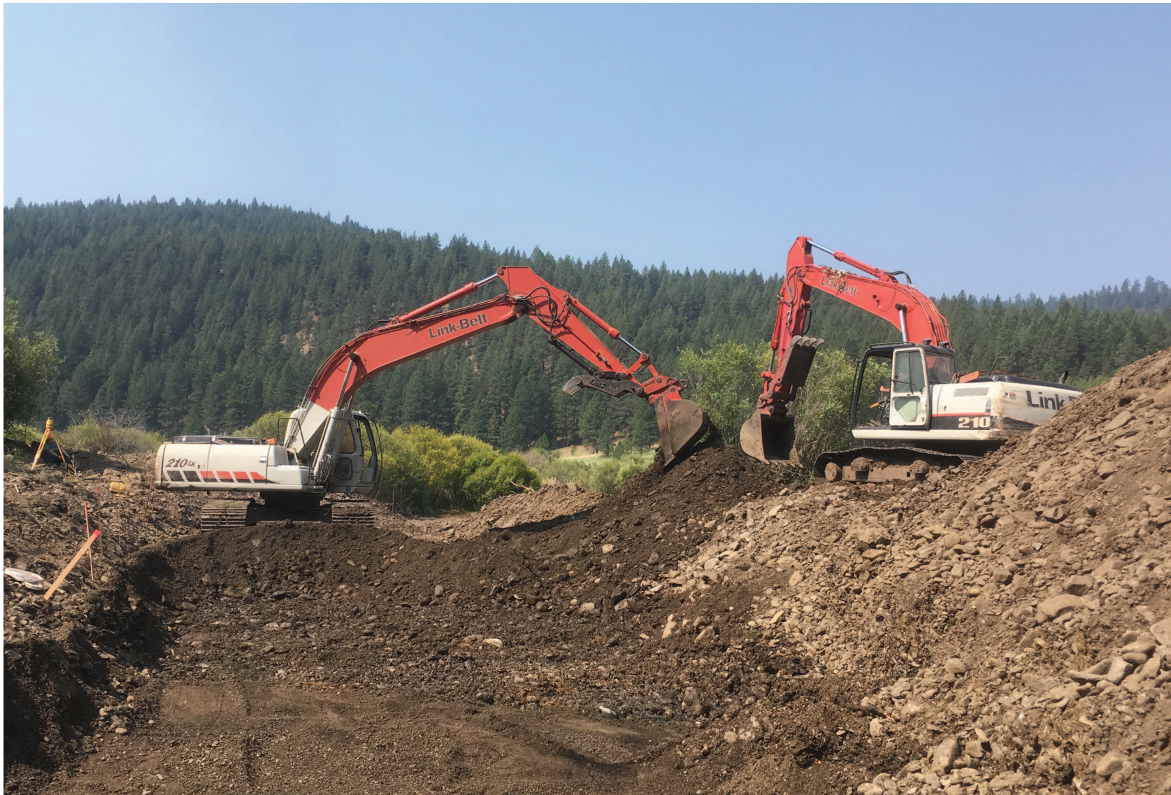
Greg and Kyle Ontko use excavators to remove historic mine tailings to reconnect Bear Creek to the Middle Fork of the John Day River near Galena as part of a 2018 fish habitat restoration project.
