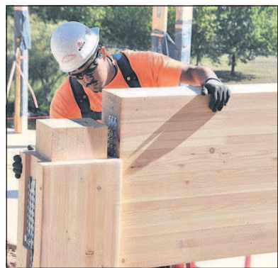
EO Media Group file photo A worker guides a glulam beam into place Oct. 3, 2017, during construction of the First Tech Credit Union headquarters building in Hillsboro.
