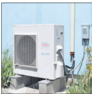
The outdoor unit of a mini-split heat pump mounted on a concrete pad on the south side of a house.
