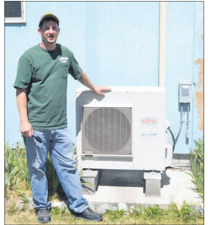
Rick Turner of MD Enterprises in Canyon City with the outdoor unit of a mini-split heat pump capable of heating a home in minus 15 degree weather.
