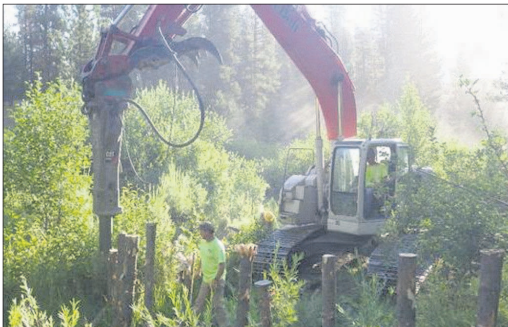
Contractors install posts that will form the backbone of porous beaver dam analogues, which will store water and cause deposition of gravels in East Fork Beech Creek.
