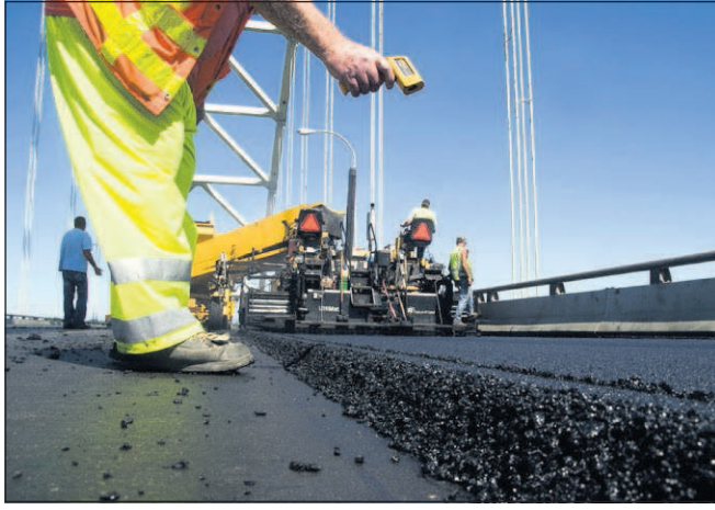
Contributed photo/Oregon Department of Transportation A crew member checks the temperature of the asphalt. Federal highway officials have warned ODOT repeatedly since 2005 that its road-paving inspection program is vulnerable to fraud.
