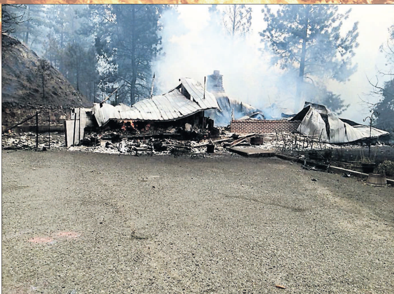
This is what was left of Dean and Courtney Fox’s home after the Aug. 14, 2015, Canyon Creek Complex fire.
