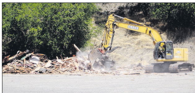
Crews demolished the building that was formerly El Cocinero Mexican Restaurant to make way for a new John Day Fire Station.
