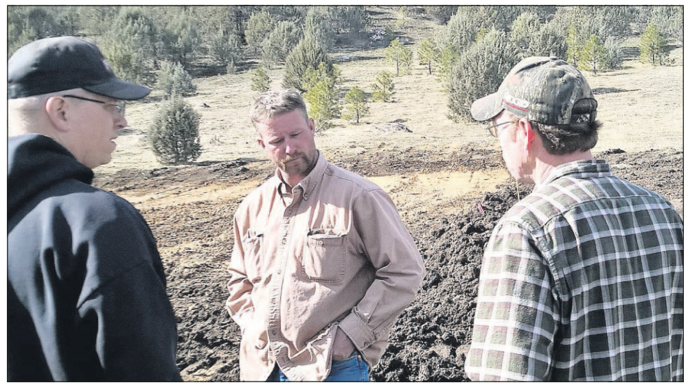
Working on the archery range at Bear Creek Shooting Range near Prairie City are, from left, Joe Hitz of Sisul Engineering, Lorin Hodge of Tidewater Construction, and Les Percy, vice president of Canyon Creek Bowhunters.
