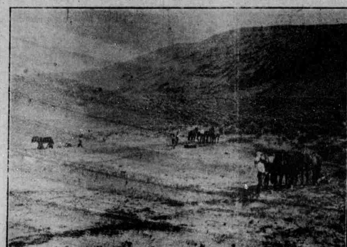
Making a Cut and Fill on the Oregon & Eastern Railroad Between here and Riverside
