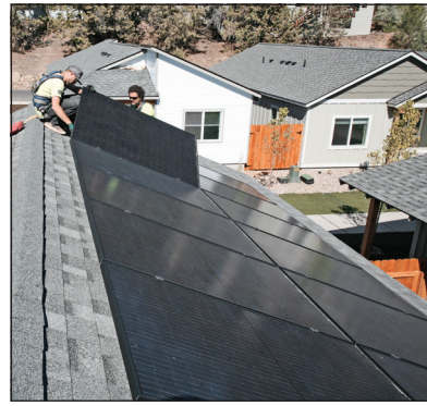
Dean Guernsey/Bulletin file Gavin Ames, left, and Travis Trondle with Sunlight Solar Energy Inc. work on solar panels on a home in Bend in 2021.
