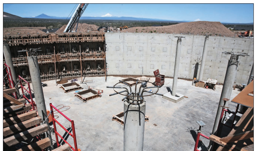
The interior of the 4-million gallon reservoir at the South Redmond Water Facility, shown here on Wednesday, will be fed by a 983-foot-deep well.
