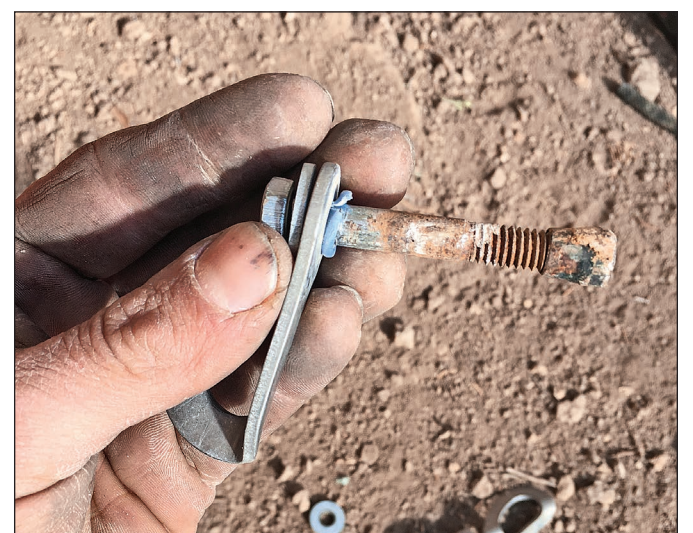
The single bolt shows corrosion at its base.
