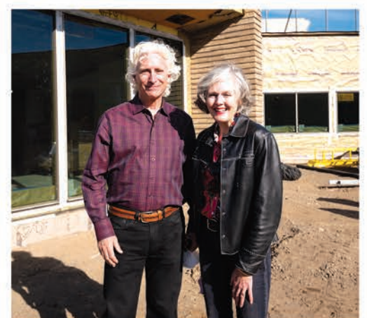
Amy Tykeson and John Teller MD recently toured the Hospice House under construction.
