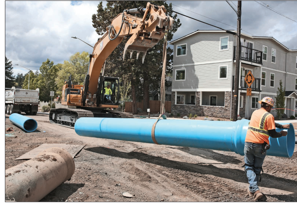
A construction crew works on a new sewer line for the Newport Corridor Improvement Project on NW Newport Avenue in Bend on Monday.
