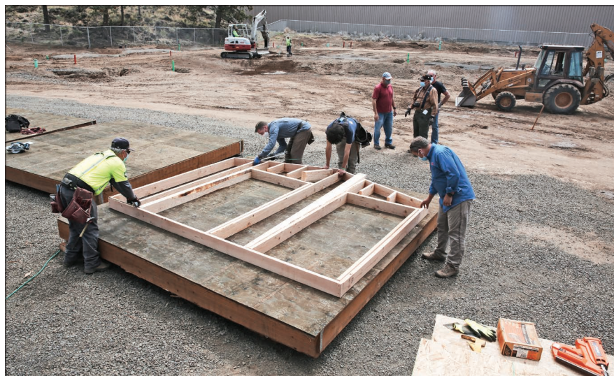
Erik Tobiason, president of Bend Heroes Foundation, right, works with volunteers and Heart of Oregon Corps personnel to build homes at the Veterans Village in Bend.
