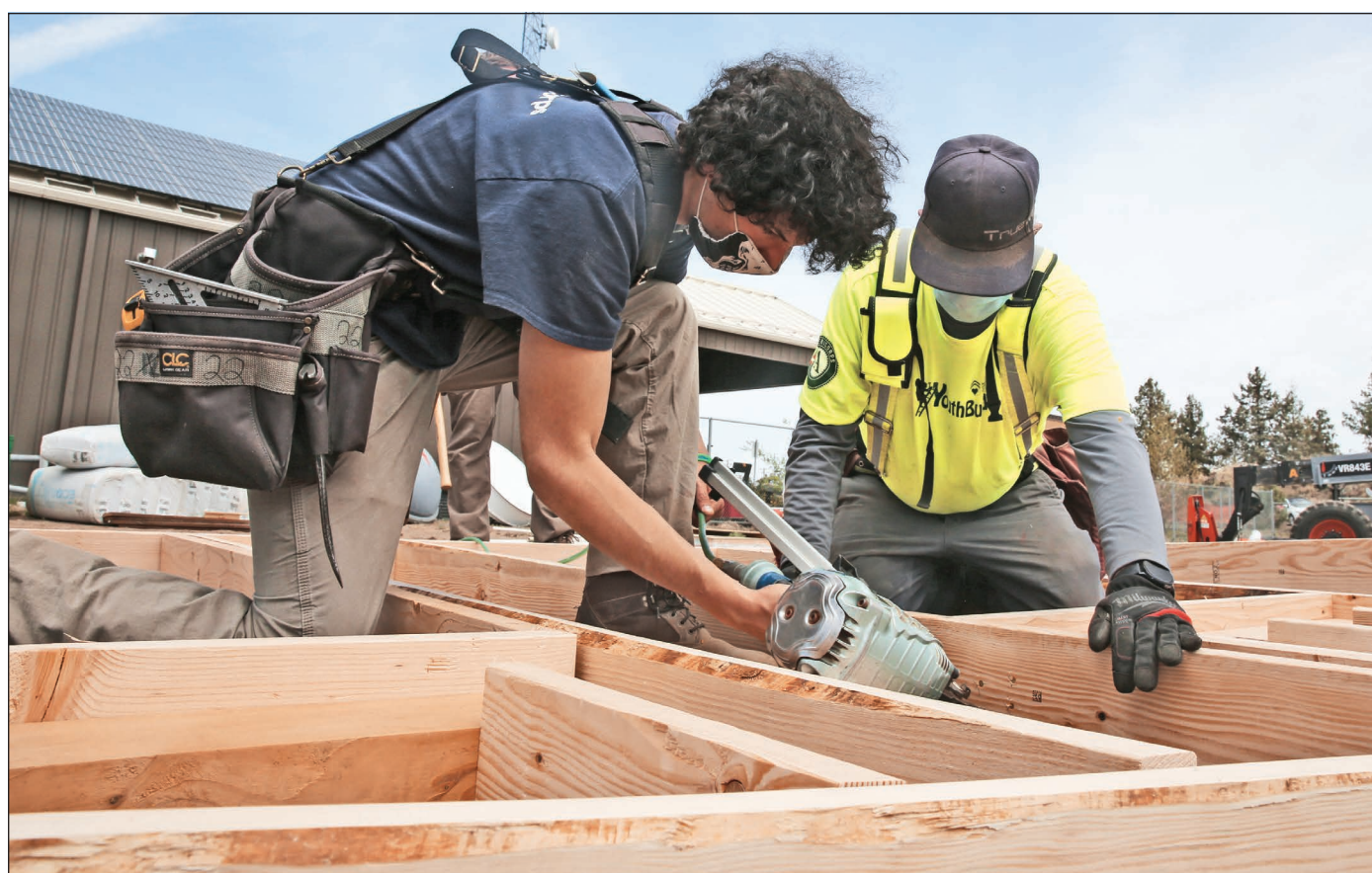
Heart of Oregon Corps Construction trainer, David Ralston, right, works with Terry Clevenger to frame a wall that will be part of one of the homes at the Veterans Village in Bend.
