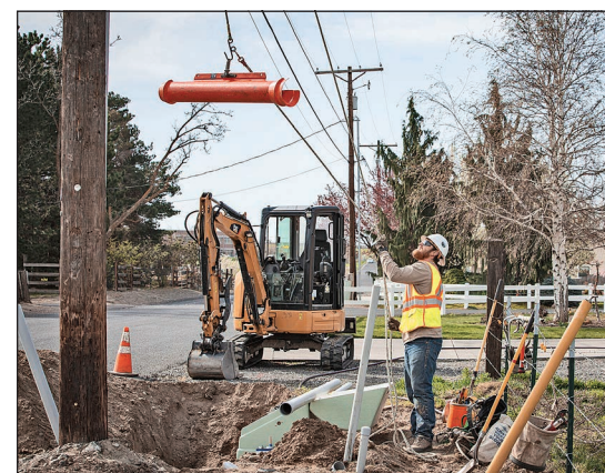
Hardie uses a rope to raise equipment up to fellow lineman Ellis while working on a utility pole in Hermiston.
