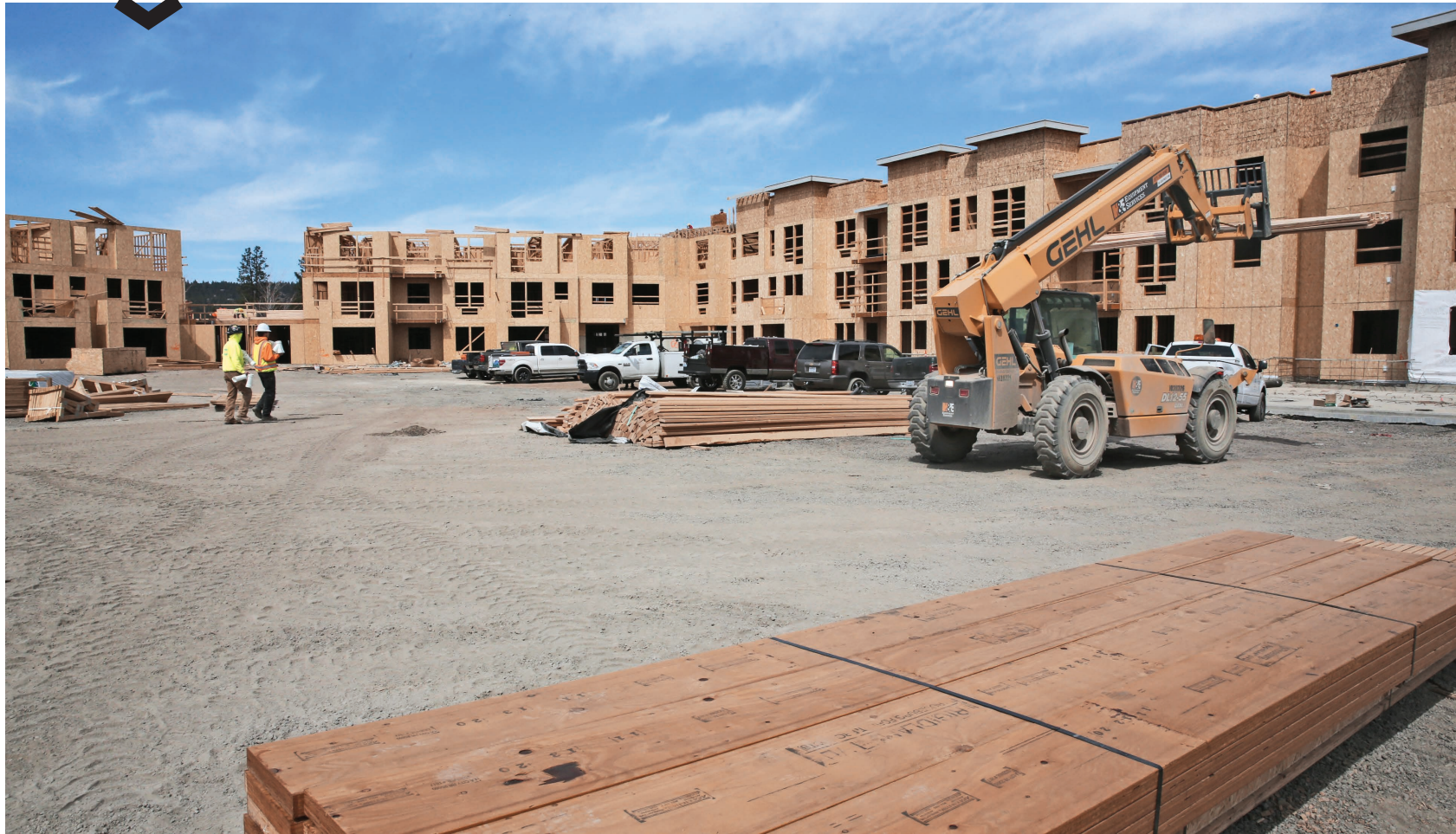
Construction continues Monday on new apartments at SW Shevlin Hixon Drive and SW Bradbury Way near McKay Park. Dean Guernsey/The Bulletin
