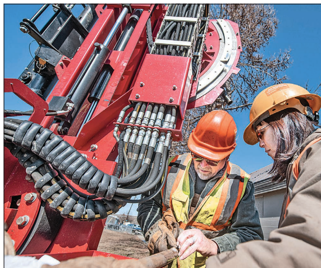
Ellen Morris Bishop/For the Wallowa County Chieftain Geotechnical drillers Michael and Marvis Remboldt on March 16 examine a core sample they drilled on the west side of the Wallowa High School Cougar Dome.
