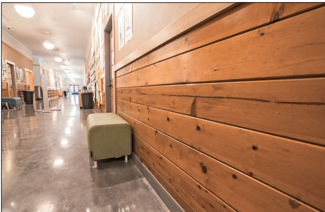
Wood paneling was salvaged during the remodel of Amity Creek Magnet at Thompson School in Bend.
