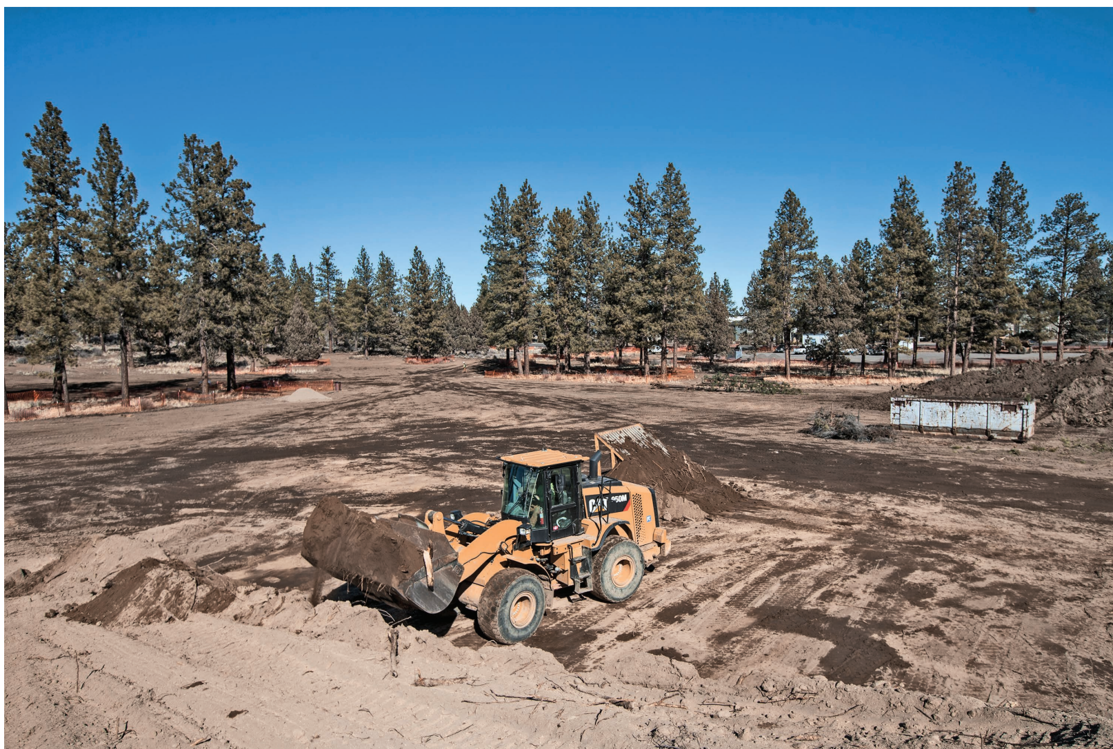
An employee of Rickabaugh Construction moves soil at Alpenglow Community Park in Bend on Wednesday. Ryan Brennecke/The Bulletin
