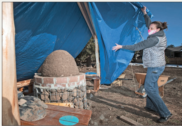
Anderson pulls a tarp back to check on the progress of a cob oven.
