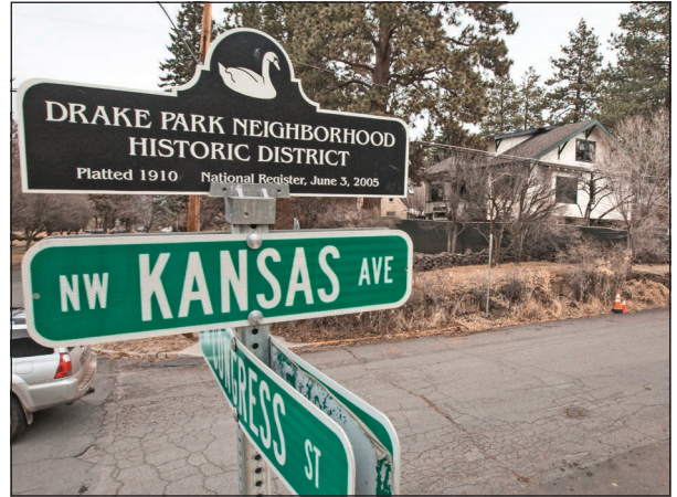
The Putnam house in Bend is raised off its foundation and is in the process of being renovated.
