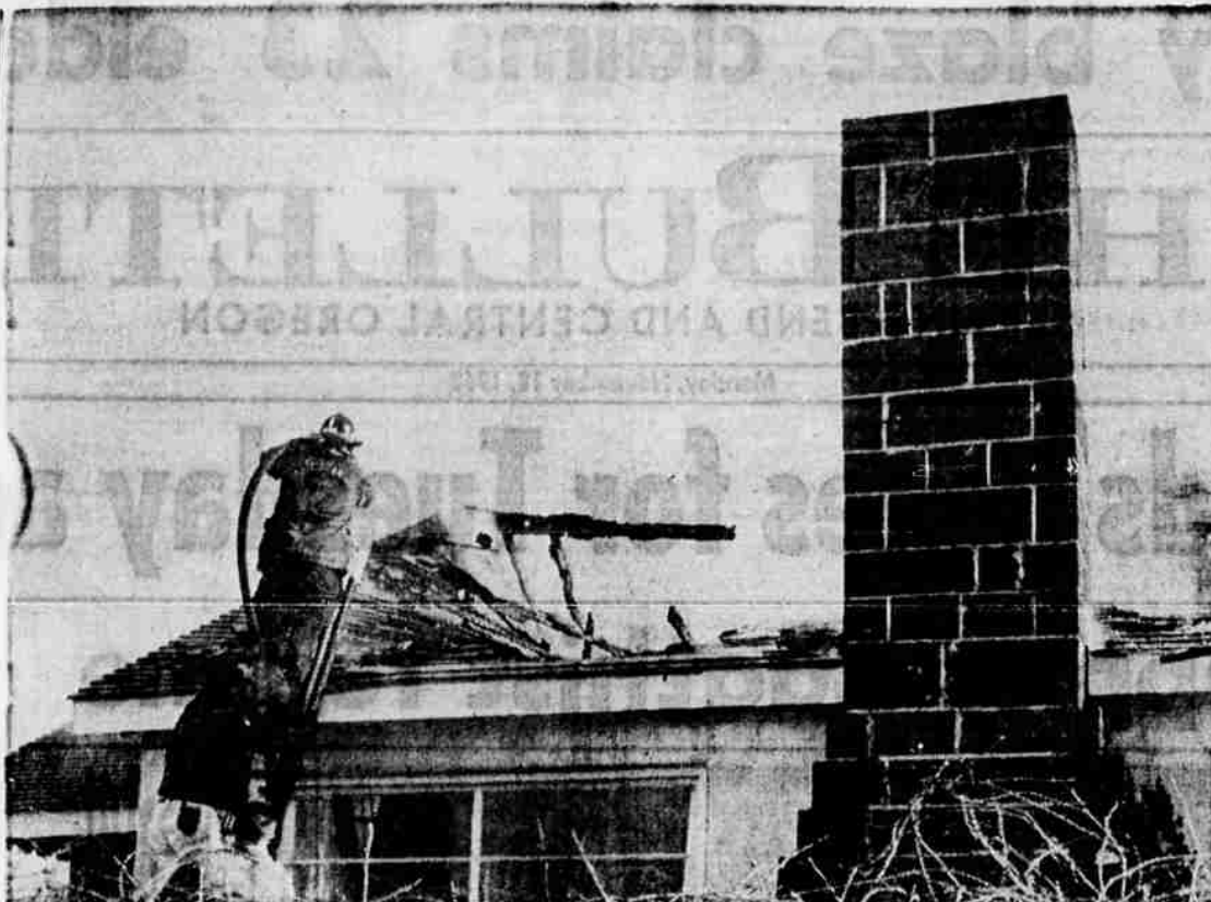
FIRE CALL — Fire of undetermined origin destroyed roof of home of Mr. and Mrs. Frank L. Kurtz, Butler Road, Saturday morning. Kurtz, on moose hunt in Canada, could not be reached and is assumed on way home. As firemen battled blaze, neighbors removed furnishings from house. Loss is being adjusted, preparatory to starting repair work.
