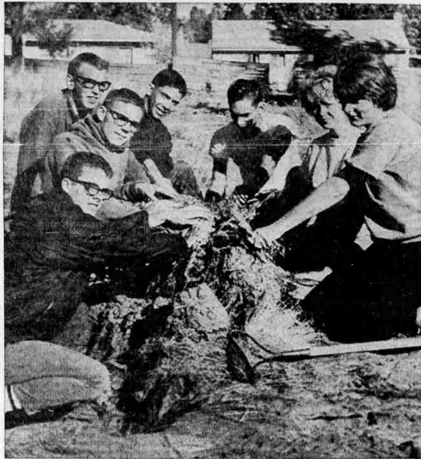
FIRST STEP — Uprooting stubborn Juniper Park stump are these members of Bend Recreation Council, engaged in preliminary work for construction of frontier-type Fort Juniper. From left are Bob Newman, Fred Raycraft, Chuck Ridderbusch, Cal Pacheco, Dennis Pacheco, Mary Ellen Dyer and Sandra Petersen.
